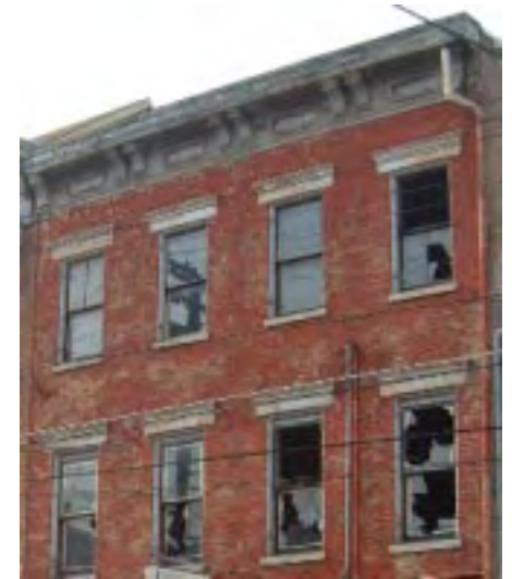
Figure 80: Broken windows in a building on Race Street. Photo courtesy of Ken Cunningham and Associates.
